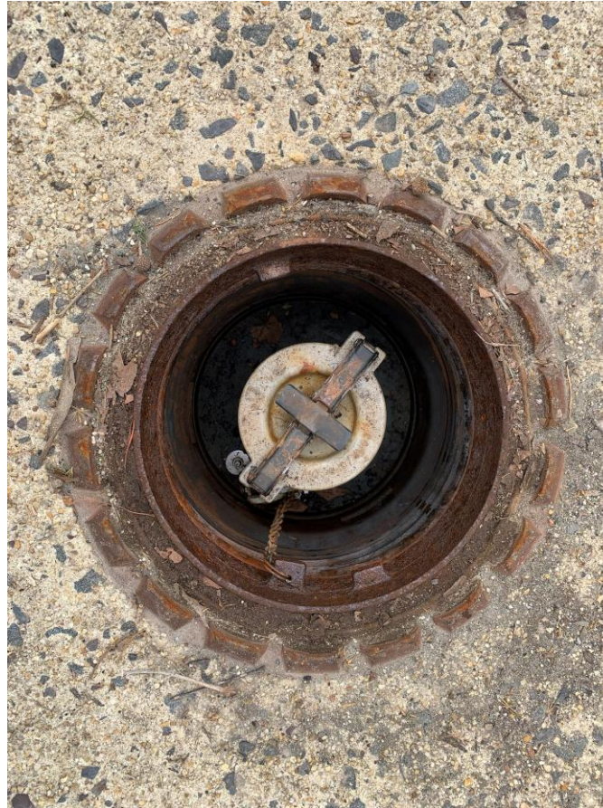
Fill Valve Spill Bucket
