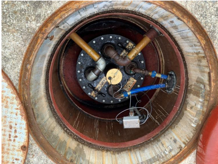
Supply Return Lines
