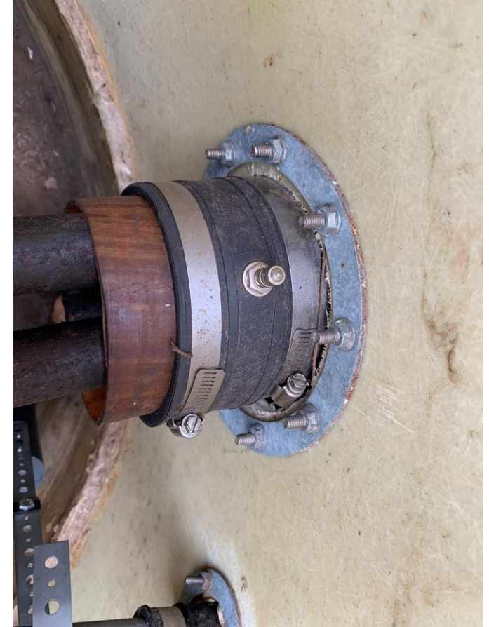
Supply Return Lines
