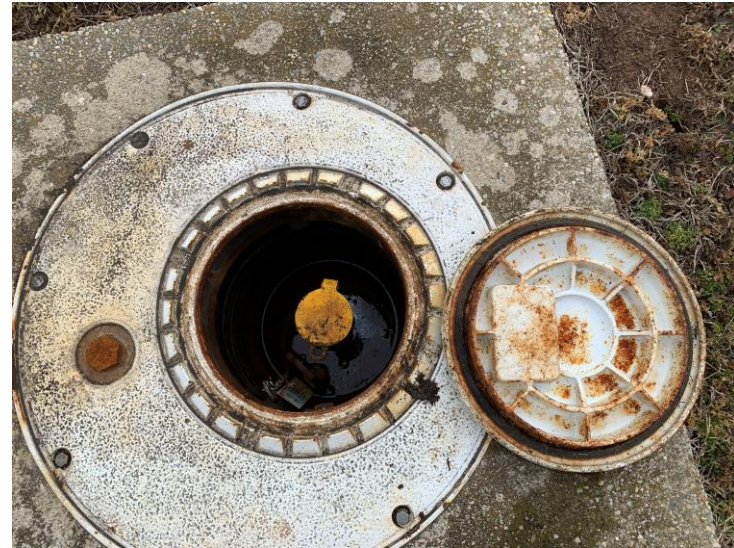
Fill Valve Spill Bucket
