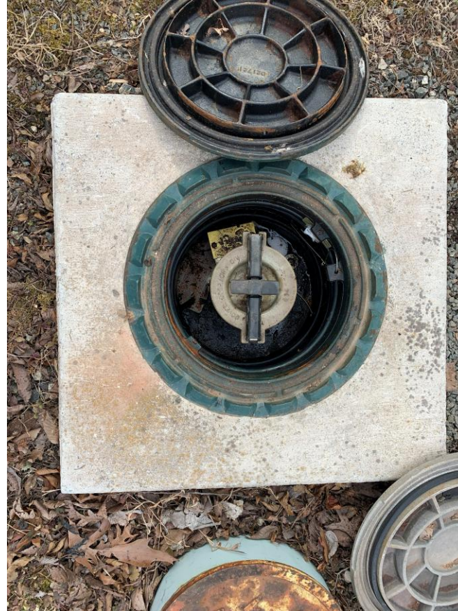
Fill Valve Spill Bucket
