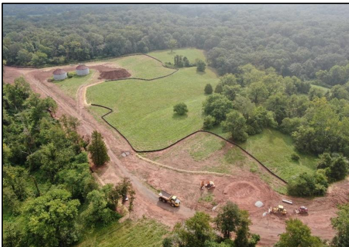
Future access road site heading northeast past existing silos. The dark line is temporary fencing being used for erosion and sediment control. It will be removed post construction.
