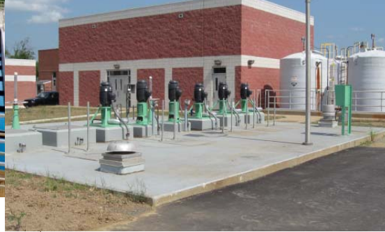
Plant Water Pump Station
