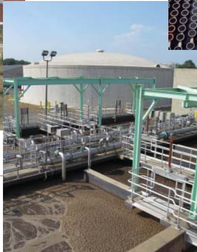
Reactor Basins (right) Reactor Basin Being Serviced (above)
