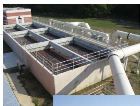
Odor Control Biofilter
