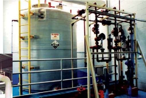
Chemical Storage Tank, Containment Basin, And Chemical Pump Feed System
