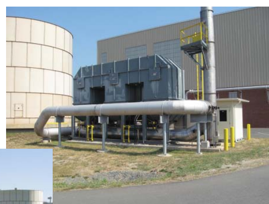
Solids Processing Building and Odor Control RTO
