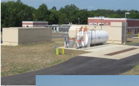
Emergency Generator and Fuel Storage Tank
